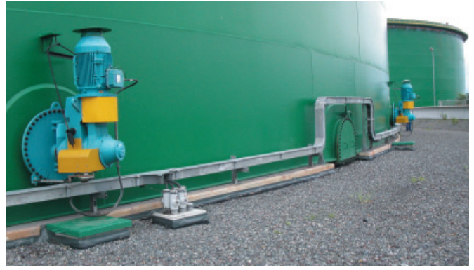
55kW Swivel Gear Mixers installed with Automatic Actuator
